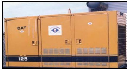
125 KW Generator Set
