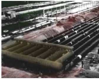
Post Weld Heat Treatment on slug catchers at the Goldboro Gas Plant.
